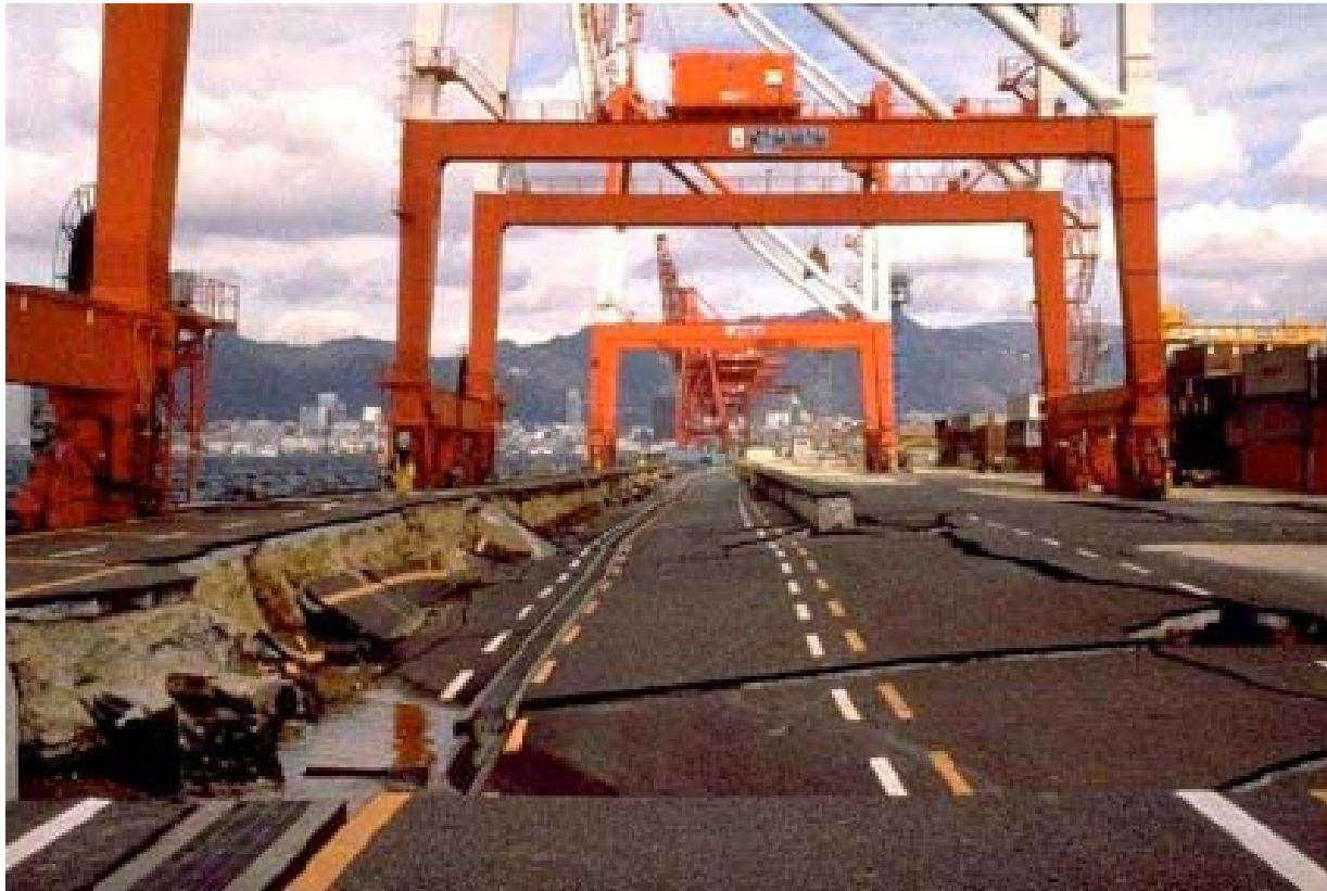
Soils at Port Island liquefied due to the Kobe Earthquake (M6.9) on Jan 17, 1995
